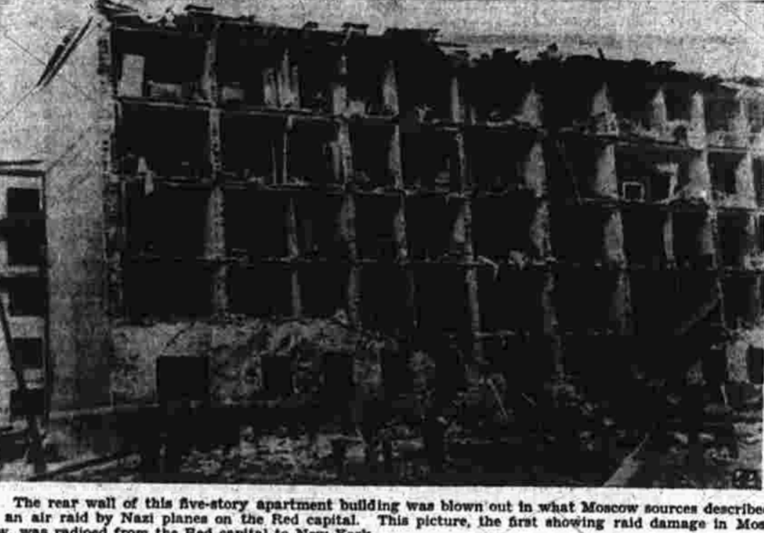
The rear wall of this five-story apartment building was blown out in what Moscow sources described as an air raid by Nazi planes on the Red capital. This picture, the first showing raid damage in Moscow, was radioed from the Red capital to New York.
